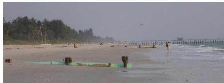
Figure 1-3. Typical Outfall Blockage (Outfall 9)
